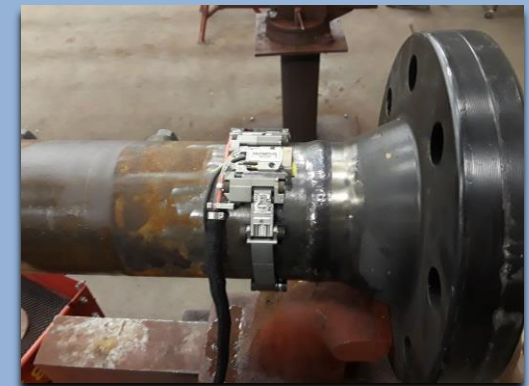
Phased Array of Process Piping
